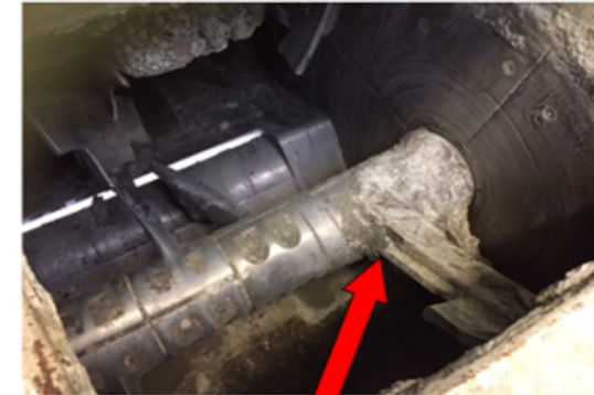
Bumped into part of the shaft to be cleaned
