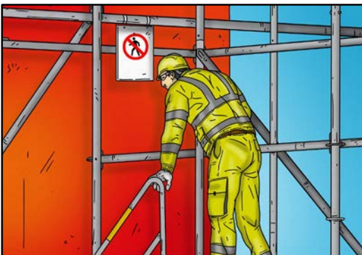
Only authorized persons can enter the scaffolding.
