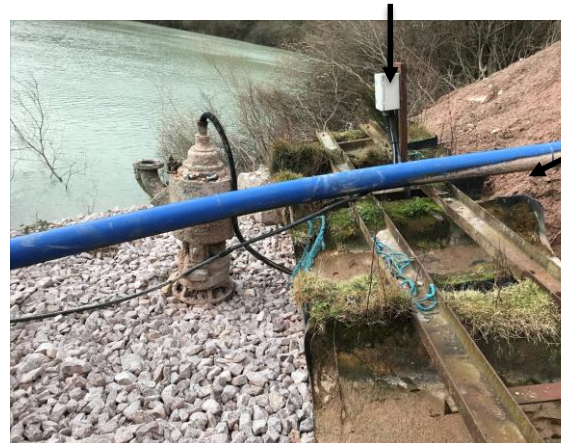
Pontoon and terminal box
