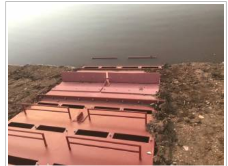
Weir Box water level control.
