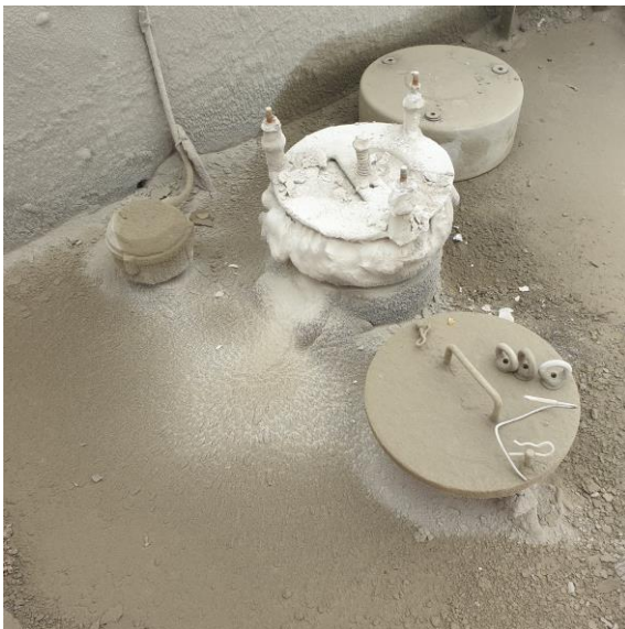
Blocked PRD – clearly in breach of permit condition but recorded as “OK”
