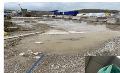
Inappropriate access route
