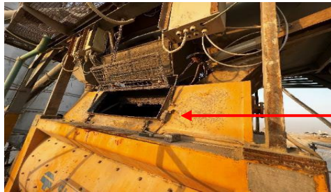
Mixer access hatch
