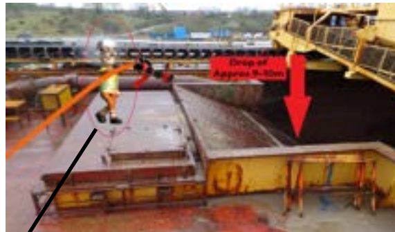
Our employee was located close to an unprotected edge
