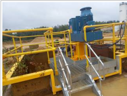
Yellow Pump Walkway
