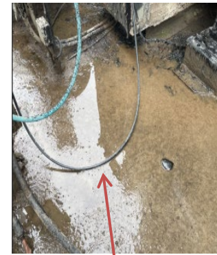
A rupture in the air pipe caused bitumen to spray upward.
